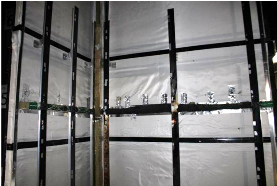
Figure 58. 3 rd full width row of horizontal cavity barriers (approx. 4800mm above chamber).
