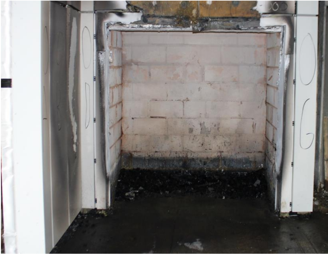
Figure 52. Combustion chamber surround.
