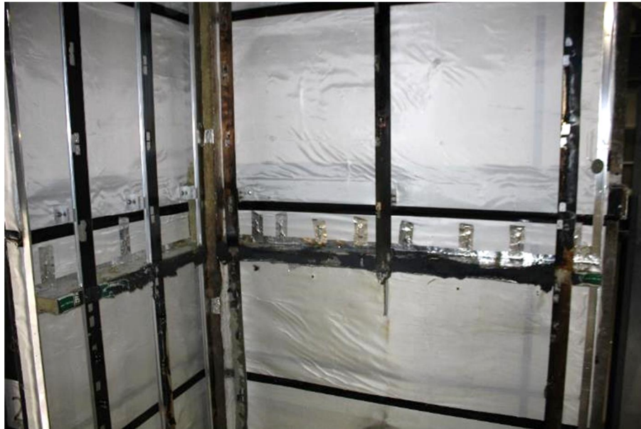
Figure 57. 2 nd full width row of horizontal cavity barriers (approx. 2700mm above chamber)
