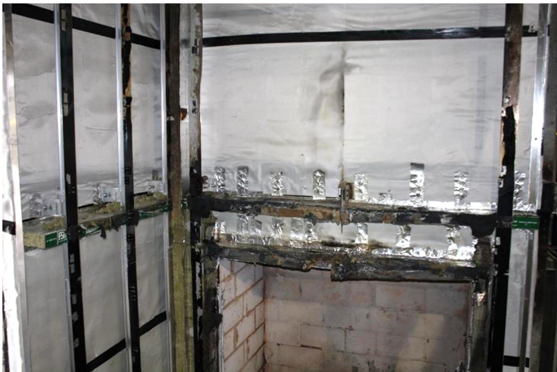
Figure 56. 1 st full width row of horizontal cavity barriers (approx. 400mm above chamber).
