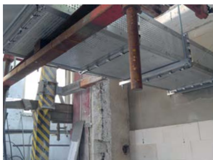
Smoke Outlet Duct
