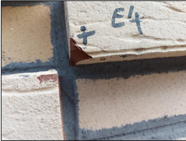
Showing damage caused following impact reference E4 on the orange zone
