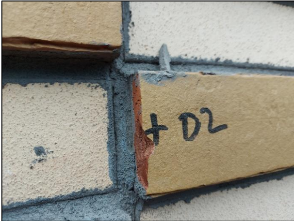
Showing damage caused following impact reference D2 on the green zone
