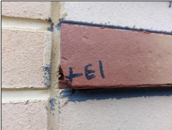
Showing damage caused following impact reference E1 on the green zone
