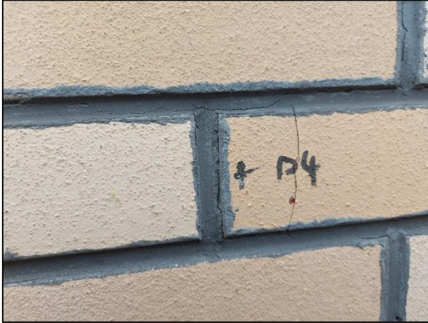
Showing damage caused following impact reference D4 on the blue zone
