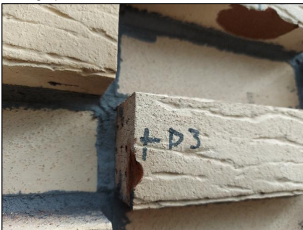
Showing damage caused following impact reference D3 on the orange zone
