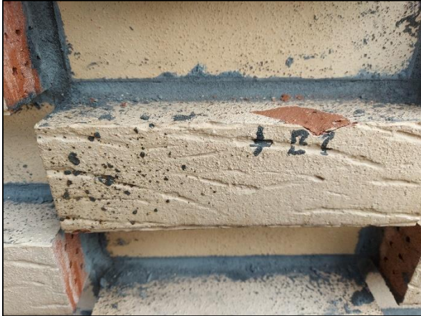
Showing damage caused following impact reference B2 on the orange zone
