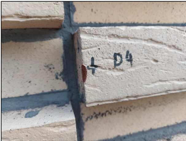
Showing damage caused following impact reference D4 on the orange zone
