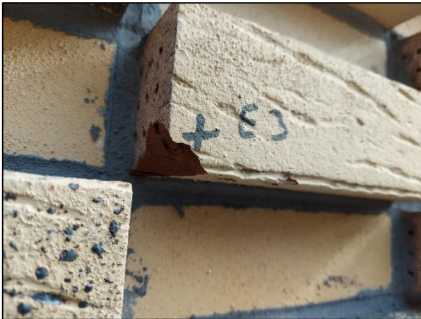
Showing damage caused following impact reference E3 on the orange zone
