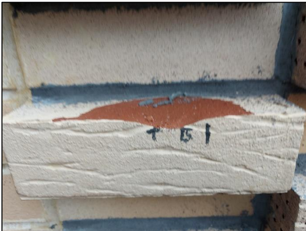
Showing damage caused following impact reference B1 on the orange zone
